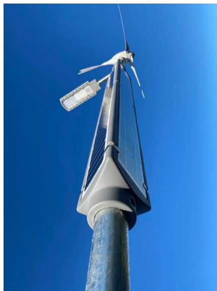
Figure 2-8 - Solar PV panel and wind turbine hybrid
